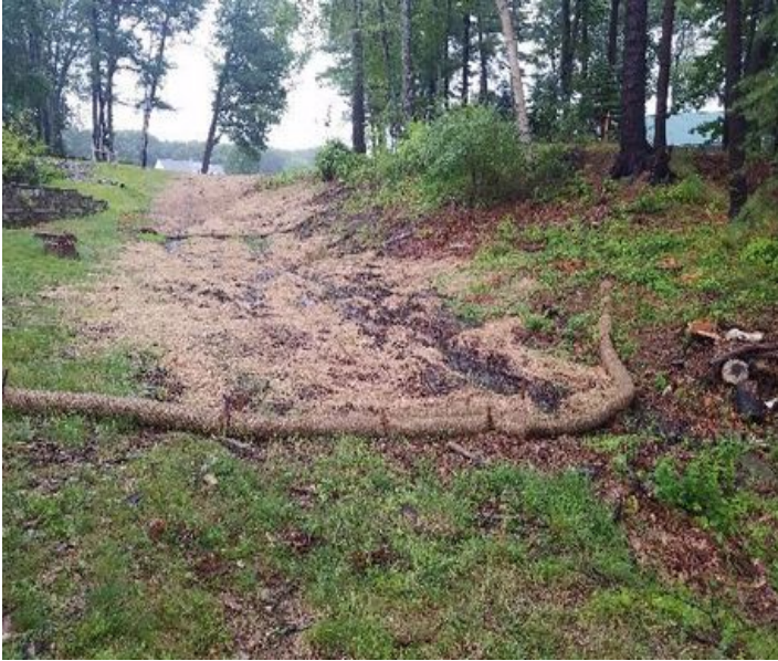
Fig 1: Gundalow Landing erosion controls, additional fence and bales are required. Viewing northeast (7-23-19).
