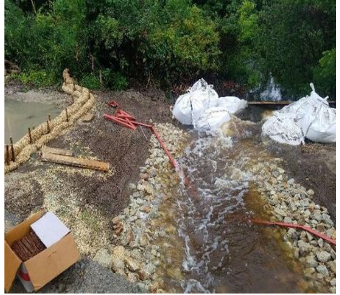
Fig 2: College Brook. High water flow due to the rain event. Viewing west. (7-23-19).
