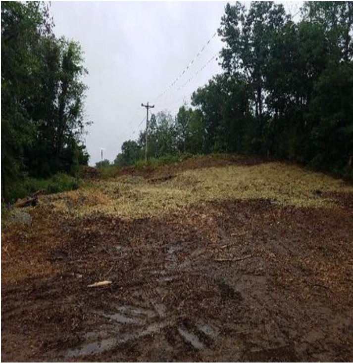
Fig 9: Area near Str. 27 where soil from Str. 23 & 24 are being spread. Viewing north. (7-23-19).
