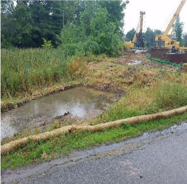
Fig 5: Wetland DW69, location of where straw bales need to be installed. Viewing east. (7-23-19).
