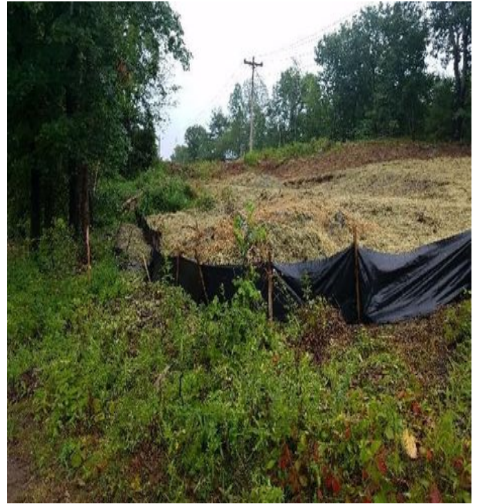
Fig 10: Silt fence installed on the downslope area of where soils are being spread. Viewing north. (7-23-19).
