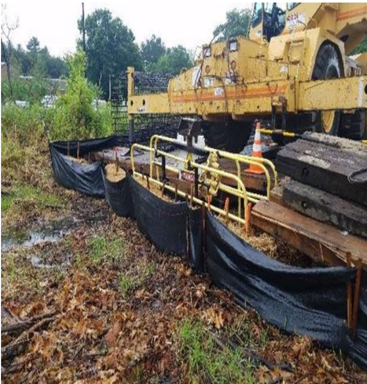
Fig 7: Erosion controls installed between drilling activities for Str. 23 and wetland DW67. Viewing west. (7-23-19).
